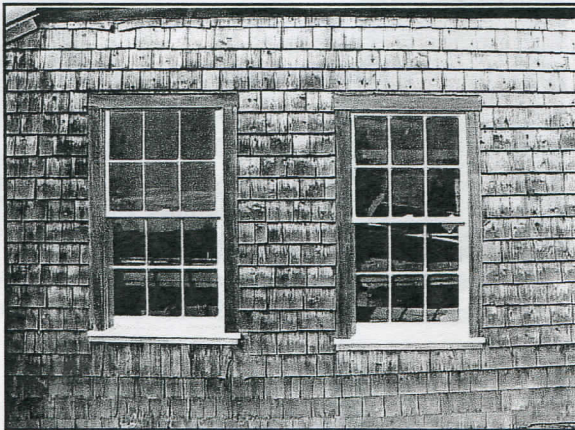
Late autumn sunshine reflected in the new windows at the Blacksmith Shop Museum. Photo by J. Battick
