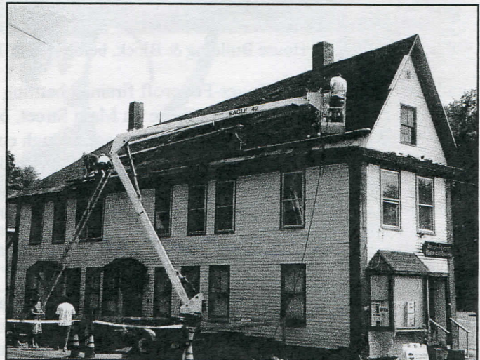
The roofing crew tackled the flat iron roof with the help of a bucket lift. Photo by J. Battick
